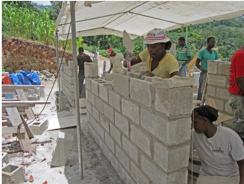
Fig. 10. Construction with Extollo: local people were trained in masonry and carpentry and employed to construct the buildings. School parent volunteers contribute to site planning and maintenance work.
